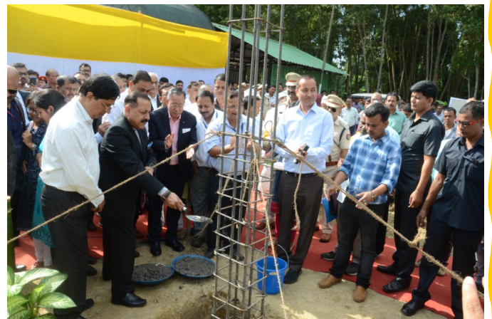
Dr Jitendra Singh, Hon'ble Minister of DoNER, laying the Foundation Stone of STINER TFC at CSIR-NEIST on 29 October 2018.
